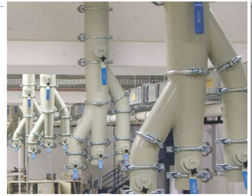
Modular pipework application
