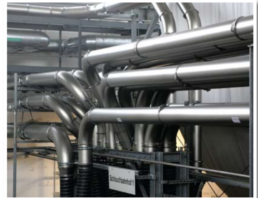
Pipework for the chemical industry
